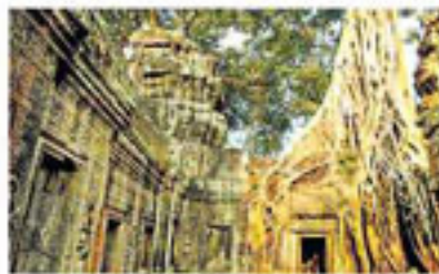
Evening at the Ta Prohm temple — the roots of the trees have taken over so strongly that it is now impossible to remove them without damaging the temple. Early morning and late evening are the best times to visit this site.
